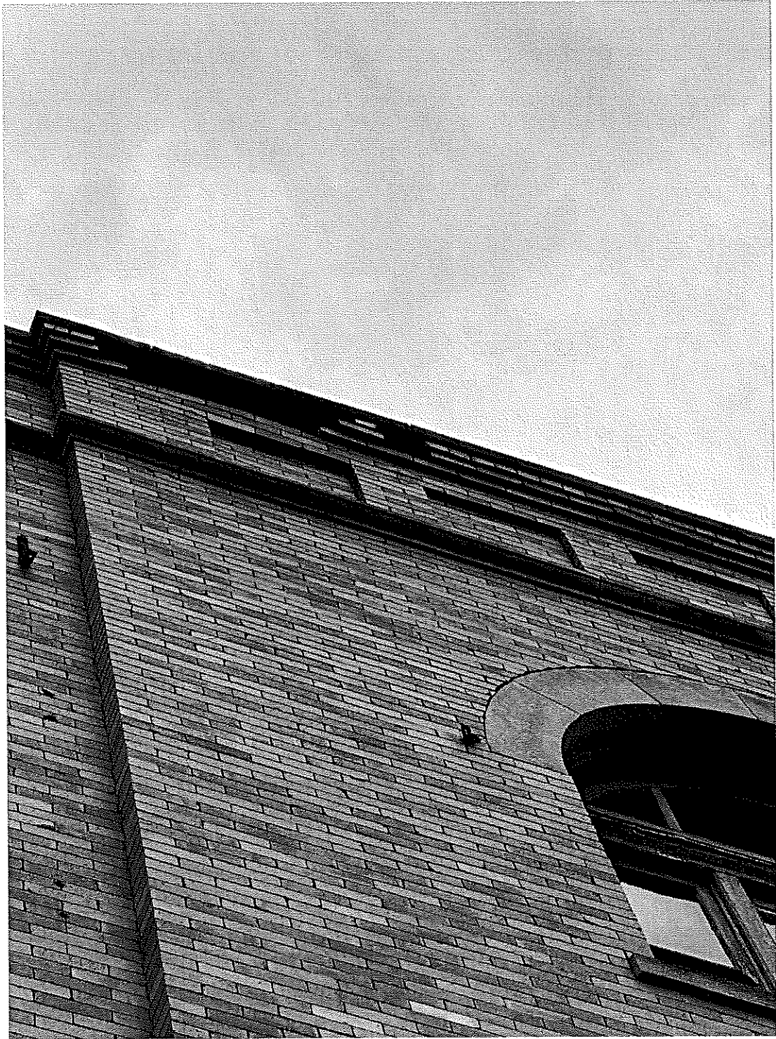
Photo 10 - Exterior Veneer at North wall, top of wall damage.
