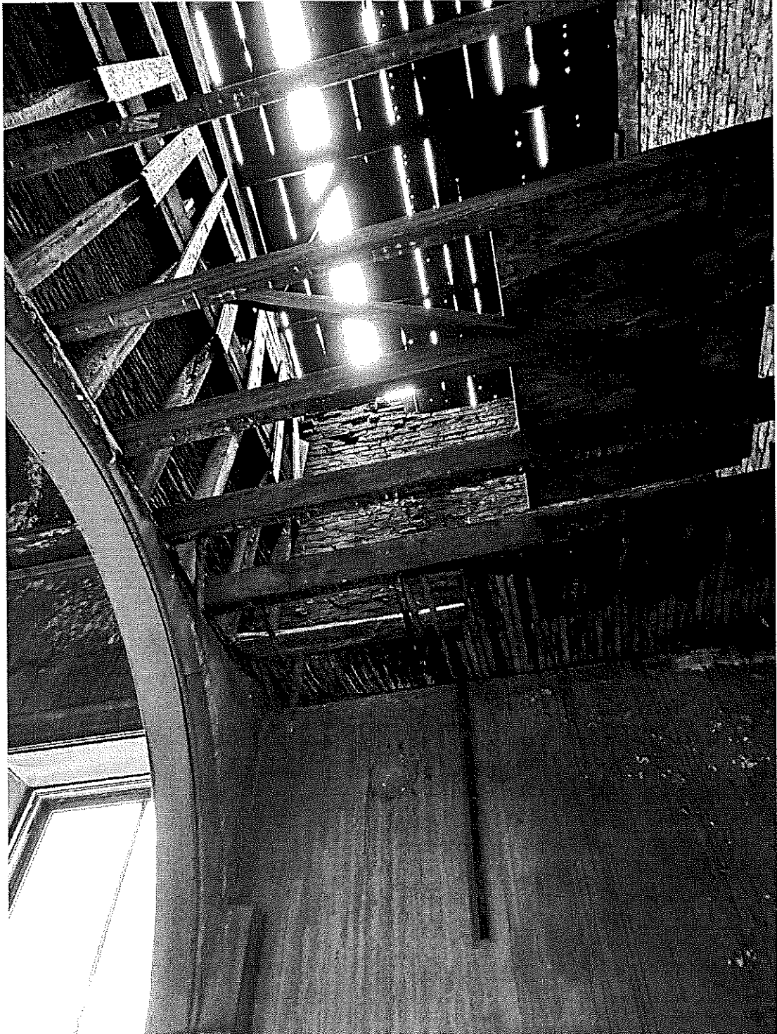
Photo 18 – South Building, south section of east wall damage.
