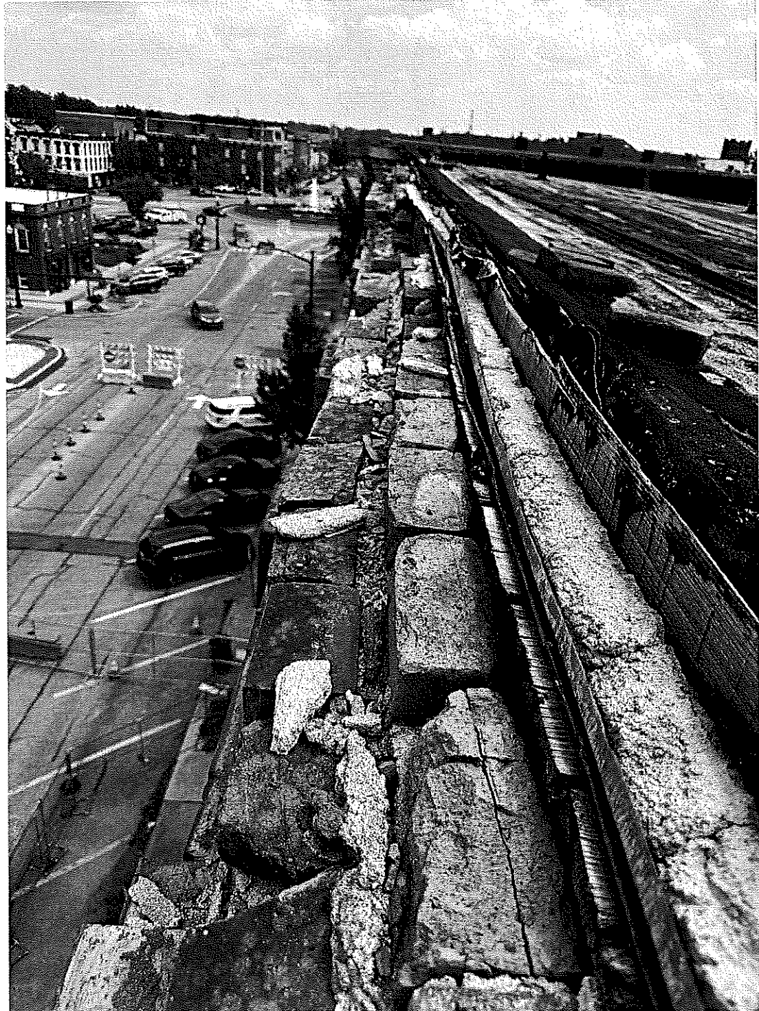
Photo 1 – North Building, North wall parapet damage looking East
