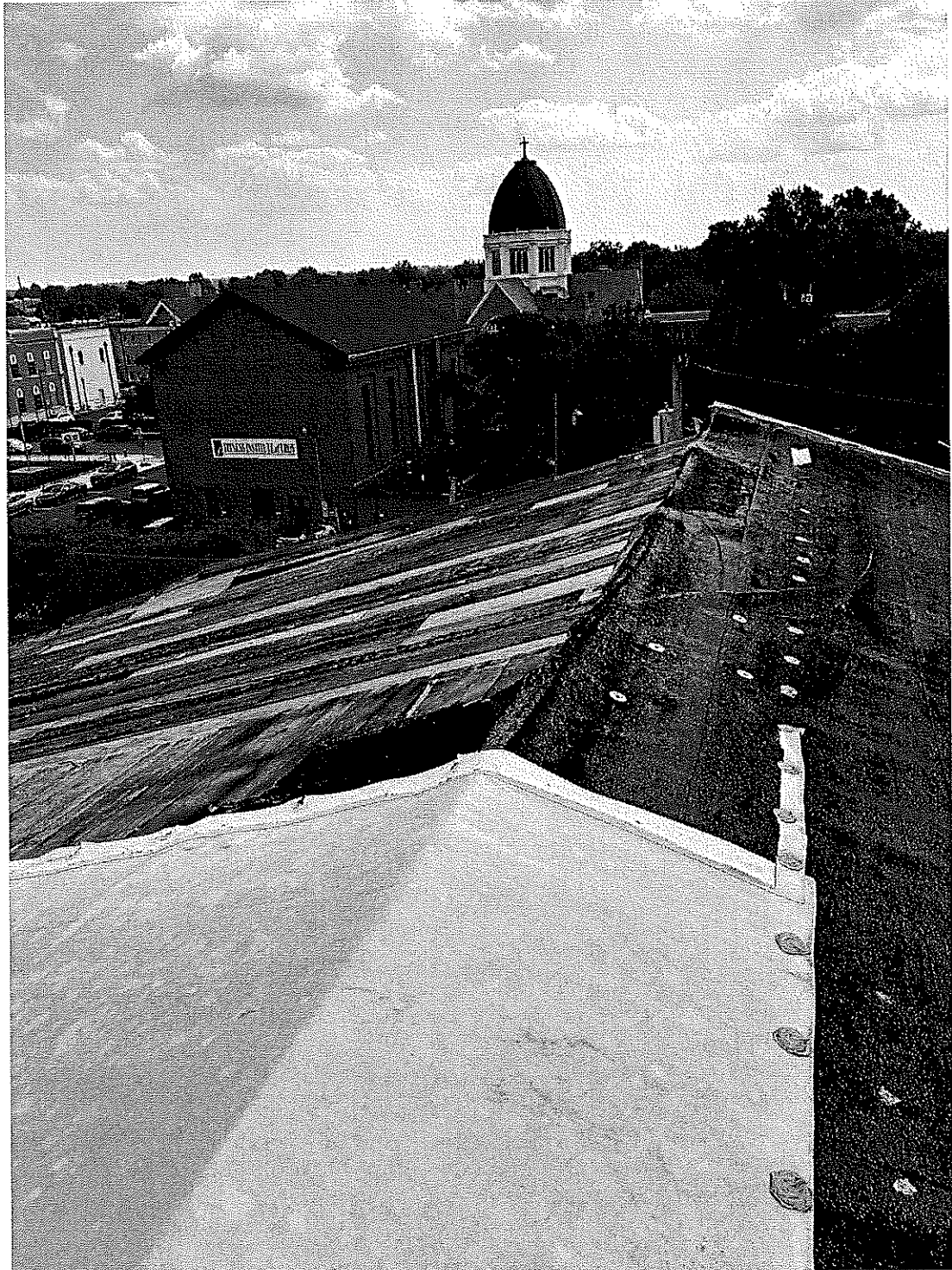
Photo 11 - South Building roof looking South at missing roofing.
