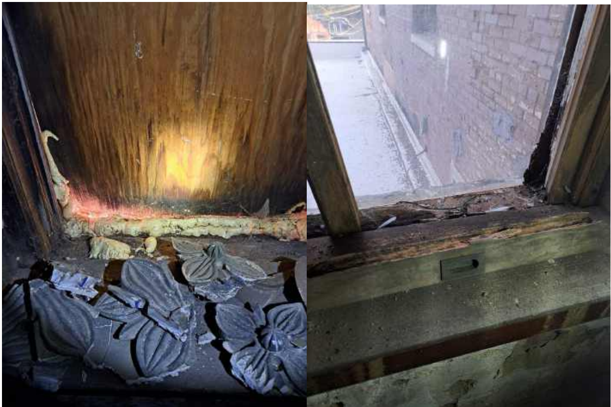
Rail of window in SE elevation (bottom of window) has rotted off
