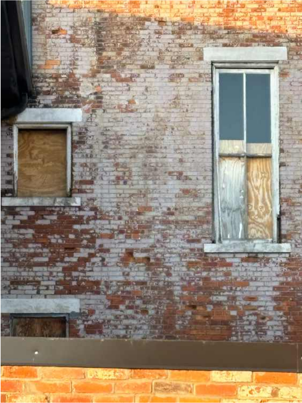
Exterior view of SE corner of IOOF building, showing window at left has been lost entirely and window at right has substantially rotted away at the bottom.
