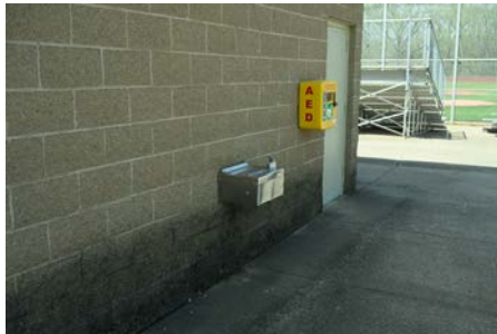
A water fountain at Duke Park should be replaced with an accessible fountain. Similar fountains are found throughout the park system.
