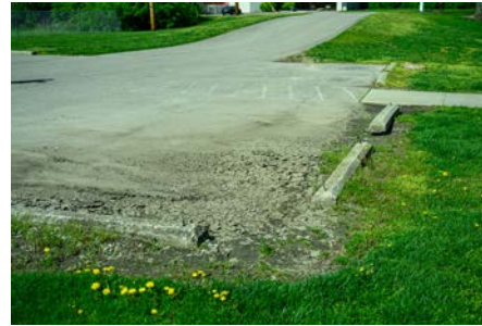
Joe Reardon Skate Park parking needs to be cleared of silt, restriped, and a van-accessible space added.
