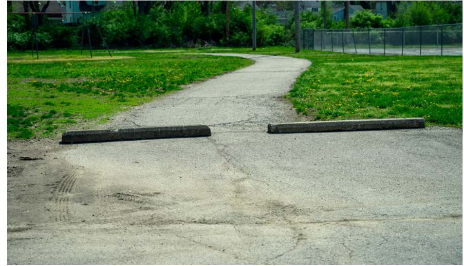
Spots labeled with the accessibility symbol at Treasure Island Park are not ADA-compliant because they should be paved.
