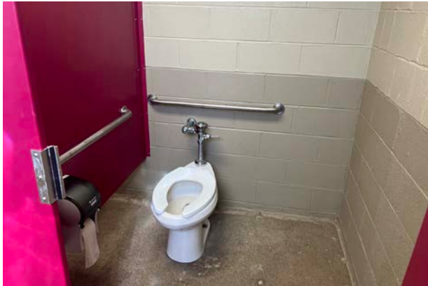
A stall at Menke Park intended to be the accessible stall should have clear floor space of 60 inches square instead of the size of the whole stall being 60 inches square. Similar stall sizes are found in bathrooms throughout the park system.
