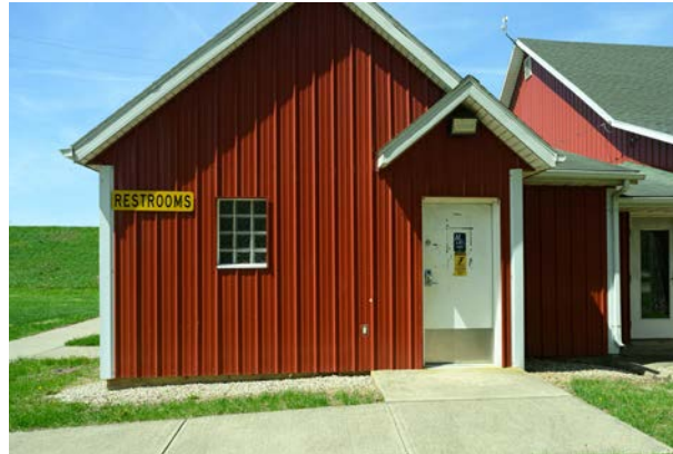
An accessible restroom at Community Park was locked in the middle of the day.
