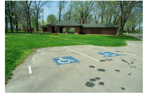
Accessible stalls at Duke Park that do not have a striped aisle to access each space, and the current aisle is not wide enough.
