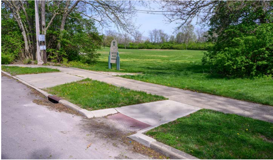
Parking bumpers at Joe Reardon Skate Park are too close together for a wheelchair user to roll between them onto the adjacent path.
