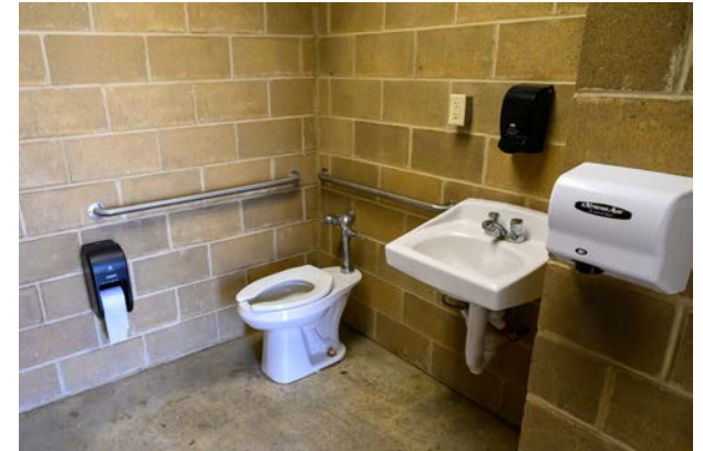
Users should be protected from touching the plumbing under the sink at Archer Park.
