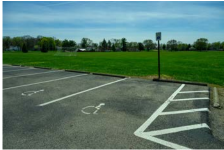
Accessible parking stalls at Community Park need to be cleared of grass with access aisles painted and at least one stall made into a van-accessible space with a sign.
