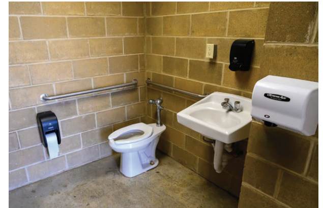
Users should be protected from touching the plumbing under the sink at Archer Park.
