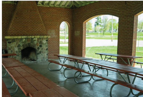
A similar situation applies to all the shelters in Community Park, where an ADA picnic table and/or a pavement connection are needed.
