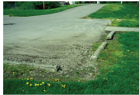
Joe Reardon Skate Park parking needs to be cleared of silt, restriped, and a van-accessible space added.
