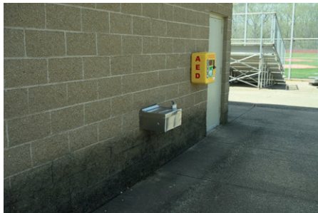
A water fountain at Duke Park should be replaced with an accessible fountain. Similar fountains are found throughout the park system.
