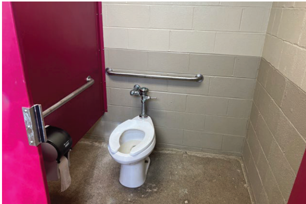
A stall at Menke Park intended to be the accessible stall should have clear floor space of 60 inches square instead of the size of the whole stall being 60 inches square. Similar stall sizes are found in bathrooms throughout the park system.
